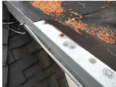
Roof edging not finished/exposed nails
