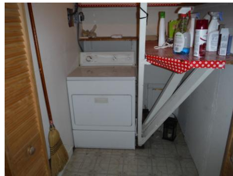
No washer hook-ups for laundry area
