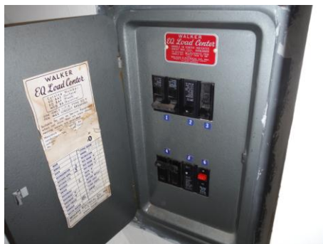
Outdated panel in bathroom
