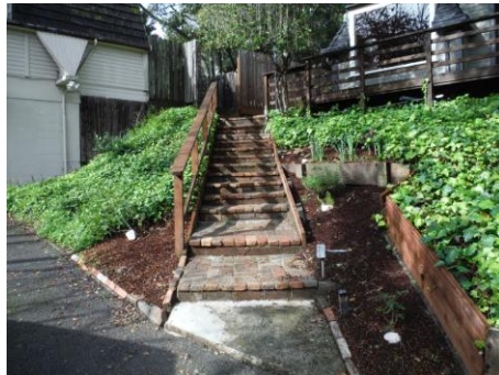
Front steps not even/railings wrong
